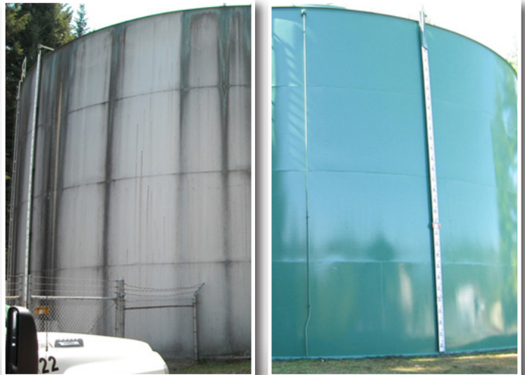
Work on the Carson water tank at Skamania, Wash., included pressure wash and lead encapsulation by applying an epoxy primer system and polyurethane top coat.
