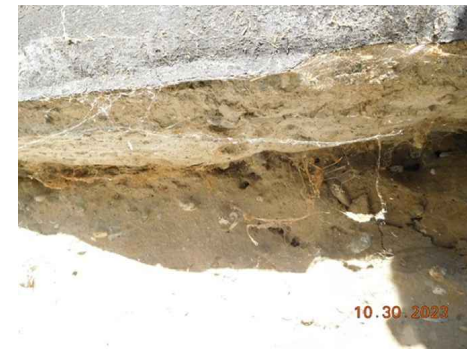
WH2B4 CONDITION UNDER RAMP EDGE
