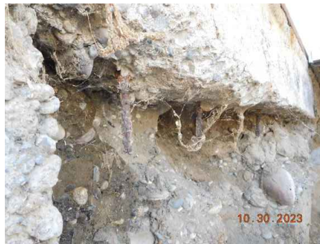
WH8B4 EXIST. CONDITION NORTH SID UNDERSIDE OF DOCK SLAB.
