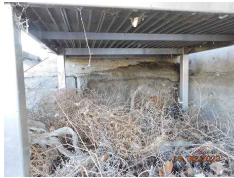
WH8B4 NORTH SIDE OF MIDDLE DOCK EXIST. CONDITION. STAIRS WILL BE REMOVED BY PORT.
