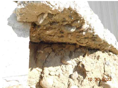
WH4B1 RAMP SLAB UNDERSIDE CONDITIONS.
