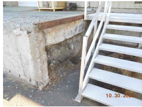
WH8B4 EXIST. CONDITION. NORTH SIDE OF DOCK. STAIRS WILL BE REMOVED BY PORT.
