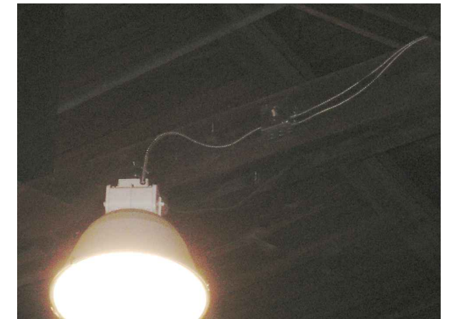
BLDG 69 TYPICAL EXISTING FIXTURE CONNECTION
