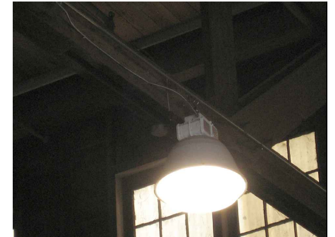
BLDG 69 TYPICAL EXISTING FIXTURE CONNECTION
