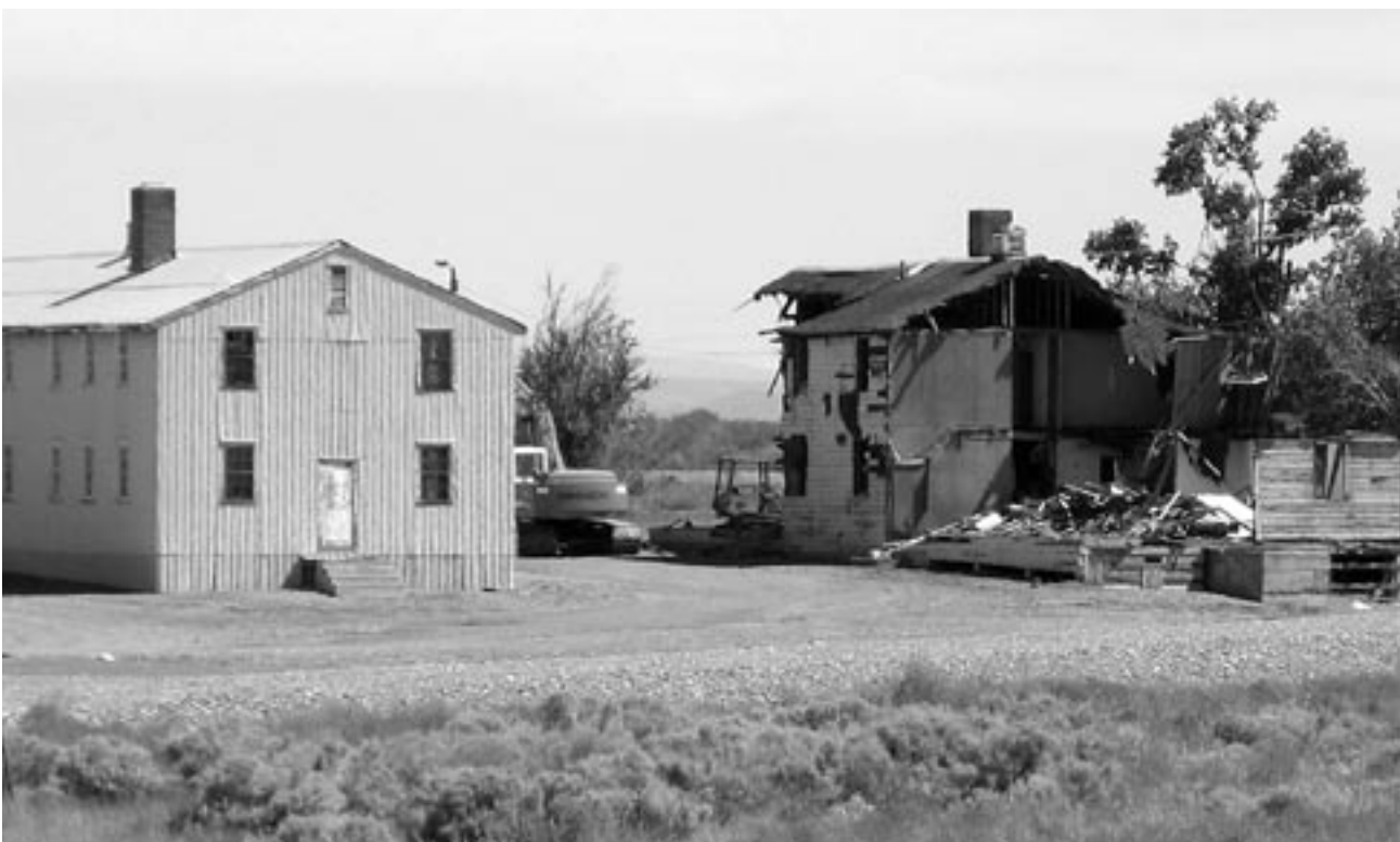
Workers remove the third of four barracks at Big Pasco Industrial Park. By the end of May, all four of the 1940s era buildings had been removed.
