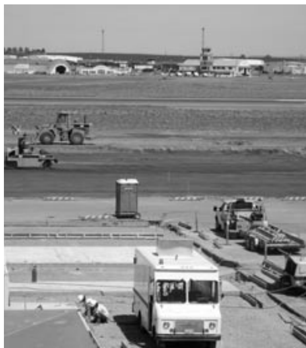
Workers are preparing the site of the new apron and taxiway. The new footprint extends the area to accommodate parking and maneuvering of the aircraft.
