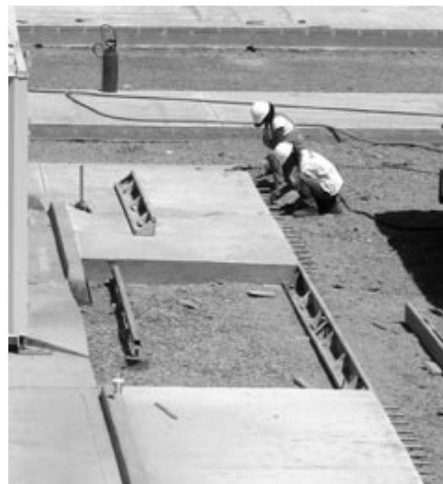
The concrete surrounding the terminal building was poured in sections. The workers inserted rebar dowels which interlock the sections together.
