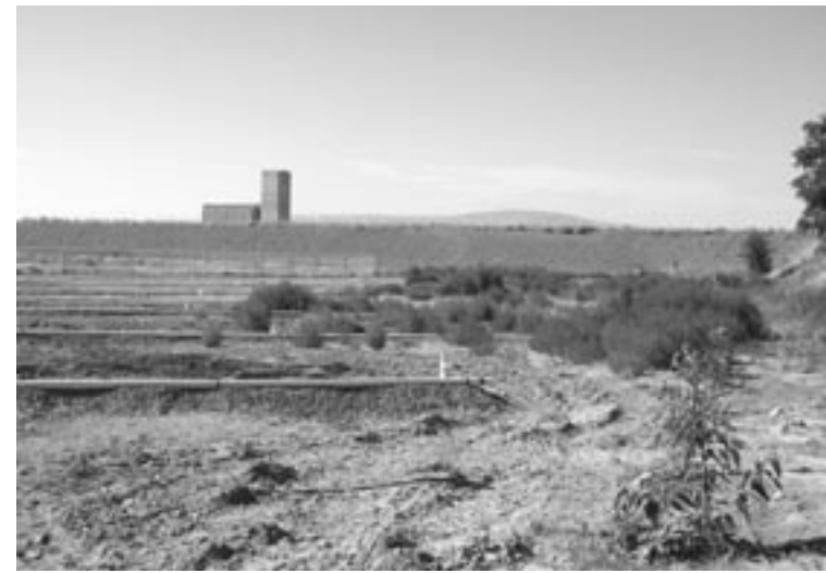
As a part of the work at the Marine Terminal site, air is forced into the ground with the use of pipes which span the site and speed clean-up.
