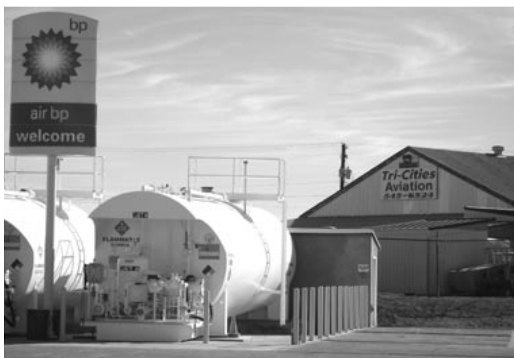
Fuel is now available to pilots any time of the day or night, with the opening of Tri-Cities Aviation. The business offers self-service fuel and has been attracting new business to the airport.
